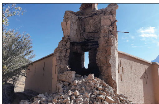
Taliban have destroyed Mohammadi's house, a resident of Sartagab village of Pato district. Local sources told the SWW that about 30 houses have been destroyed in Sartagab, Biri wa Barma villages. /Photo by: Mohammad Raja
