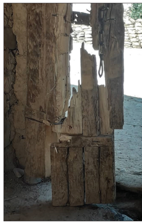
The door of Moradi's house broken due to the Taliban's raid at Moradi's house. Photo by: Local source
